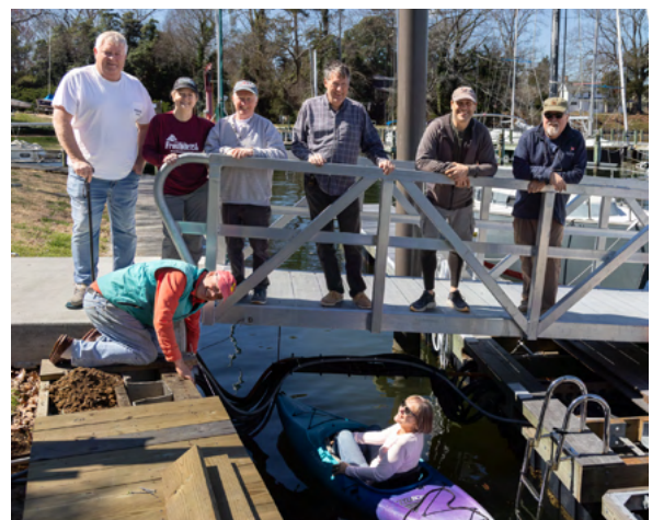
Club WiFi installation on the Docks!
